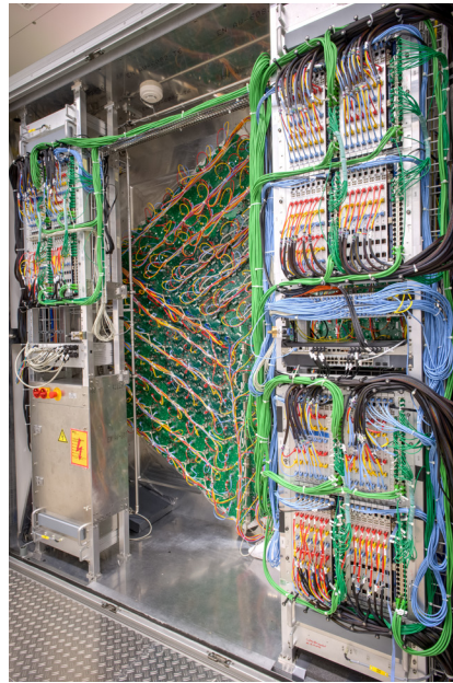
Rear view of FlashCam with electronics units and cabling.
